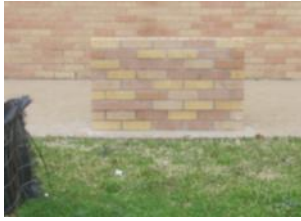
A sample wall is constructed on the left to determine if the new bricks will match the old.
