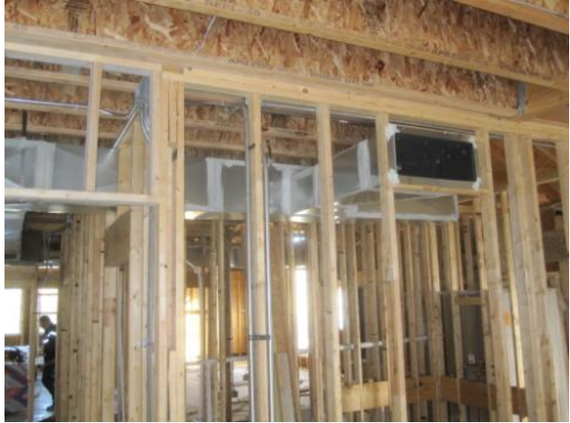
Duct work, plumbing, and wiring is added to the interior of the “Cube.”
